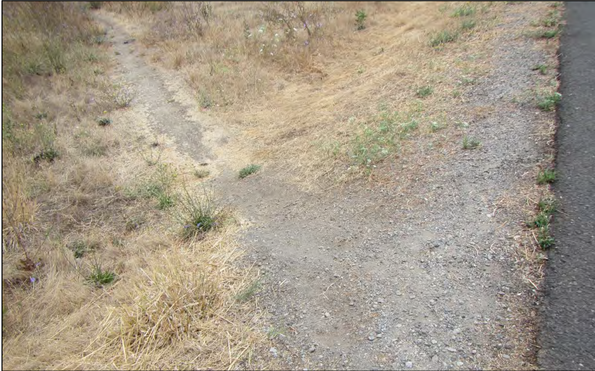
Figure 5-2: Inspection Point NLT3_2020_a_0011: Rutting along the levee slope
