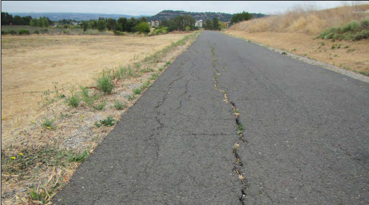
Figure 5-3: Inspection Point NLT3_2020_a_0020: Cracking observed in asphalt
