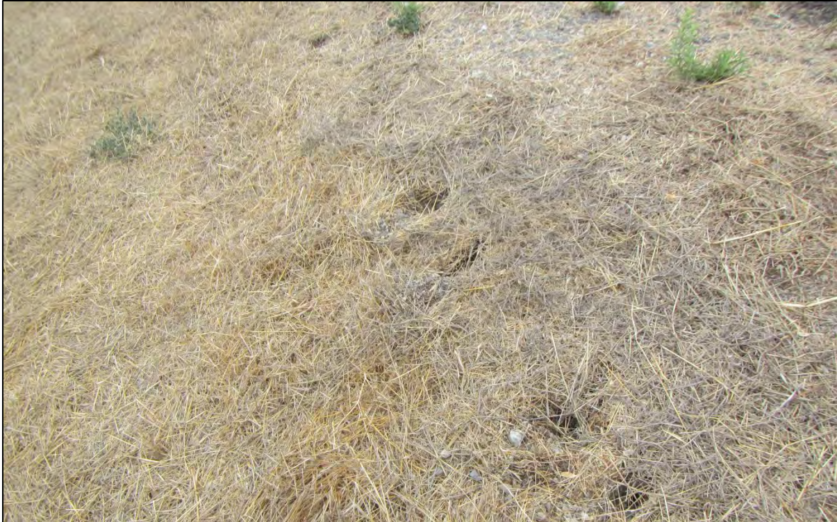
Figure 5-4: Inspection Point NLT3_2015_a_0020: Animal burrows on the downstream slope of the levee.
