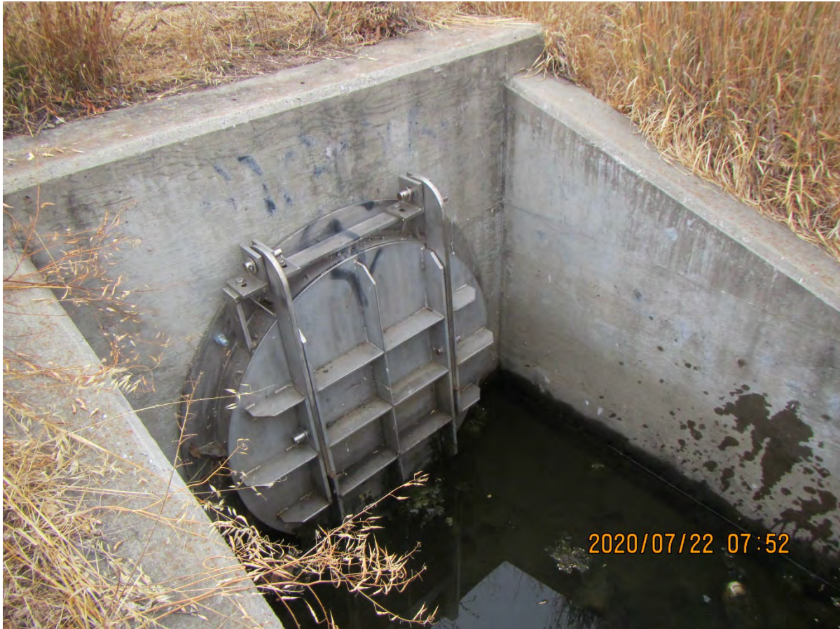
Figure 5-5: Inspection Point NLT3_2015_a_0008: Headwall structure and flap gate on the Caltrans Drainage Structure
